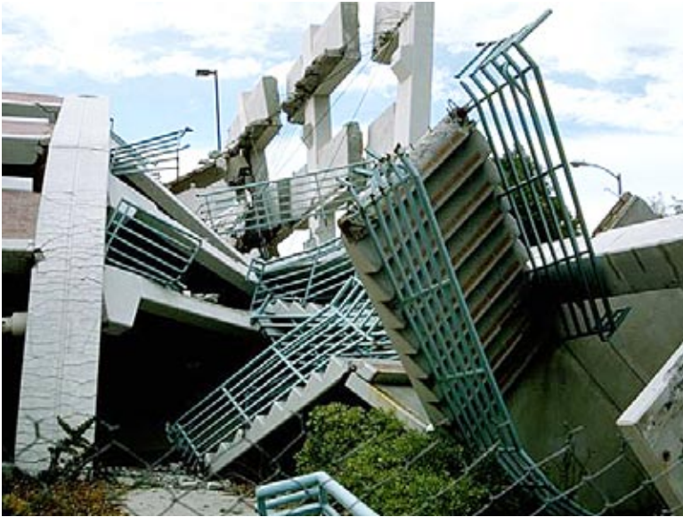
An earthquake destroyed this building.
